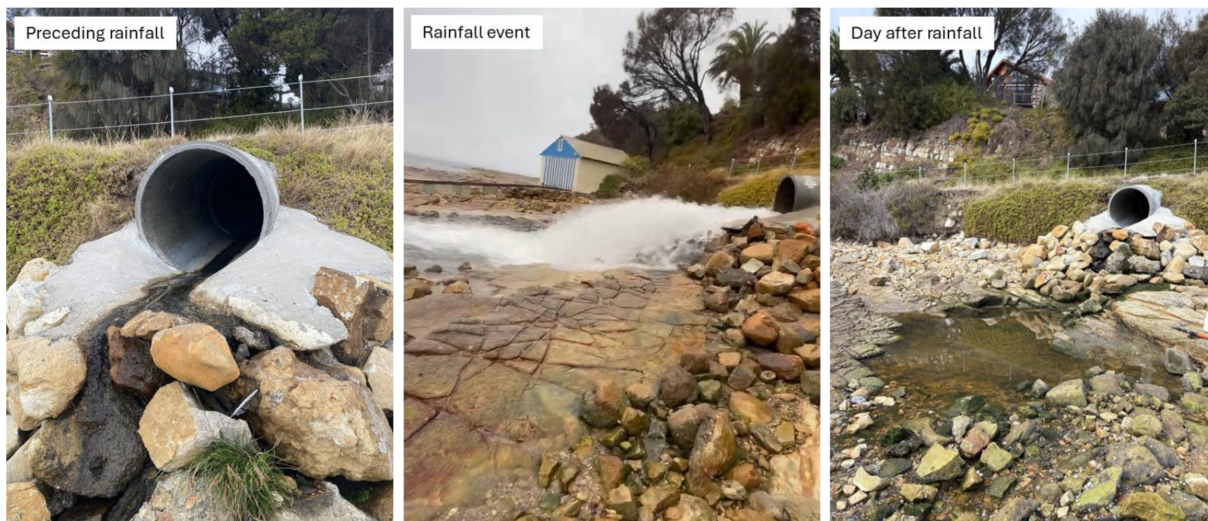
Figure 19. Conditions at the Flowerpot stormwater outfall and rockpool below during the March 2026 water quality sampling event, showing trickling discharge preceding rainfall (on 23 March 2026), high volume discharge during rainfall (24 March 2026) and trickling (minimal) discharge again after rainfall (26 March 2026).
