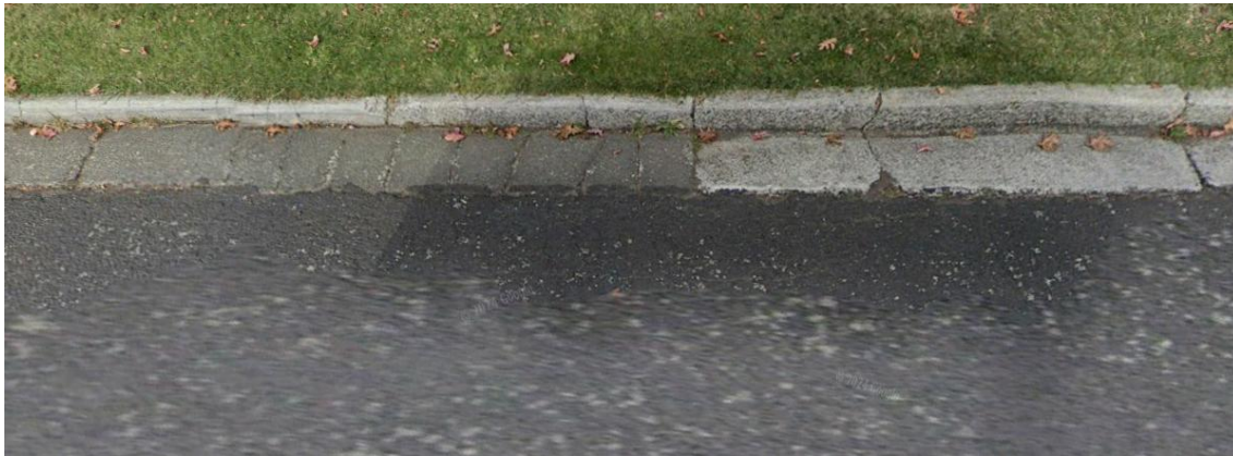
Figure 2: Cracking in the current drainage; image from Google Street View
