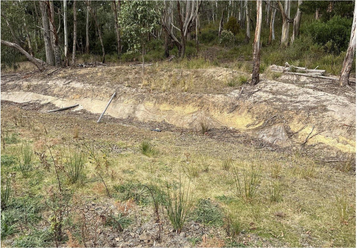
Photo 3 Exposed cut batter at the rear of the upper bench, showing previous excavation into soil/weathered material. This cut forms part of the uncontrolled earthworks assessed for stability.
