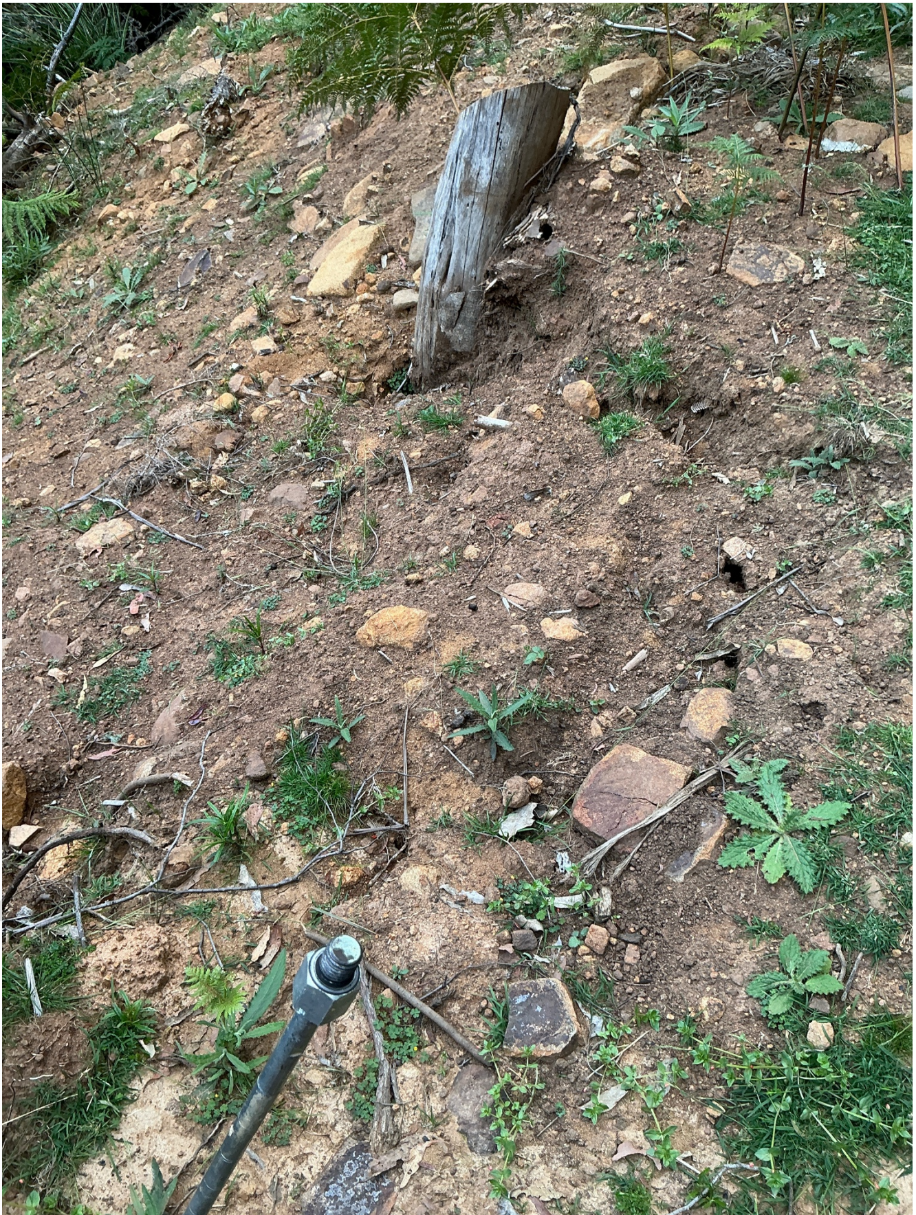
Photo 6 Evidence of tension cracks within the road fill in this section of the driveway.
