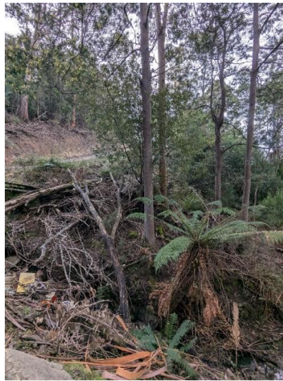
Figure 5.2-2 The first corner of the access track will require widening to meet BAL requirements, likely by 'filling in' the inside of the corner which is within the Waterways and Coastal Protection Zone. The existing culvert may also need replacement.
