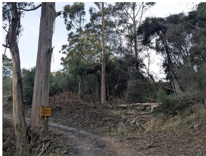
Figure 5.2-3 The third corner of the access track will require widening to meet BAL requirements, by clearing a small amount of vegetation on the outside of the corner. The culvert under the track may also need replacing which is within a Waterways and Coastal Protection Area and close to the base of a Very High Conservation Value Eucalyptus globulus .
