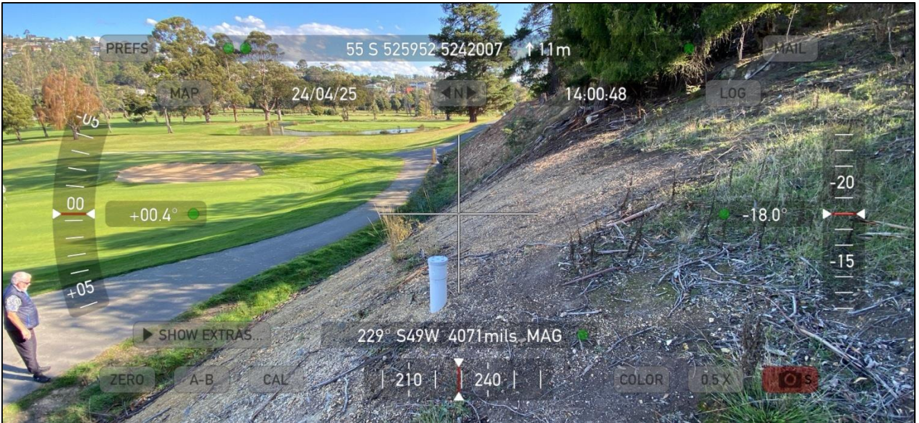
Figure 20 - Alignment of new sewer line where Tree # 11 was removed (just right of centre)
