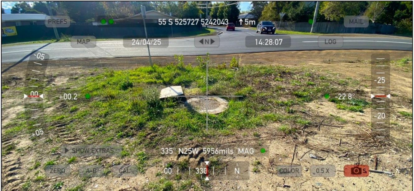
Figure 31 - Alignment of new sewer line where it crosses the Channel Highway to join the pre-existing sewer network
