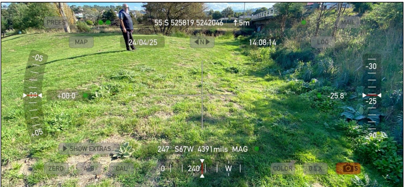
Figure 26 - Location where drilled line under Browns River emerged (approximately 20 m from rivers edge)
