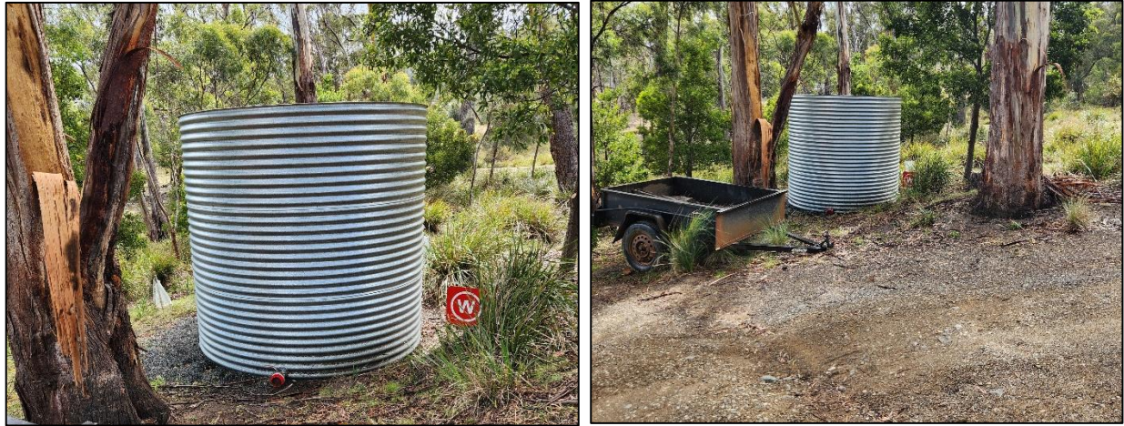
Photos 11 to 12 – Existing 10,000 L firefighting water tank with compliant signage and fitting located within 3 m of hardstand driveway and approx. 8 m to Apollo Bay Road.
