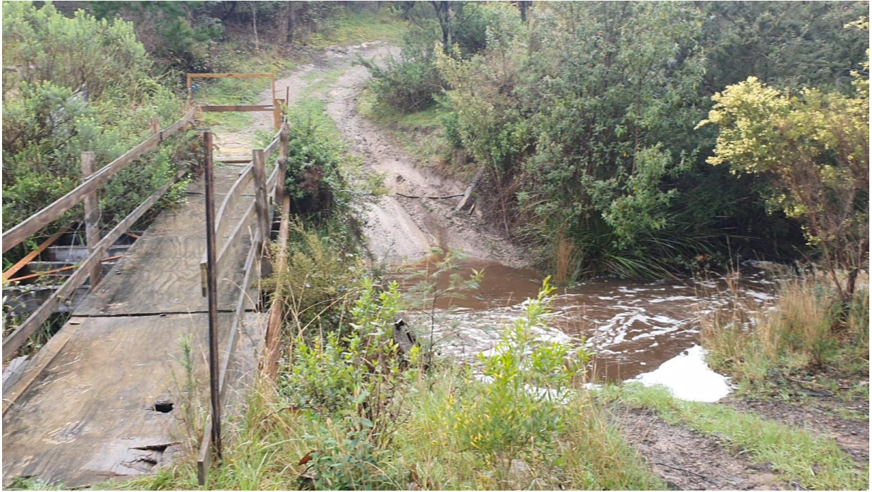
Plate 1. View of bridge prior to replacement showing bypass with muddy exit/entry points [© C. Weir]
