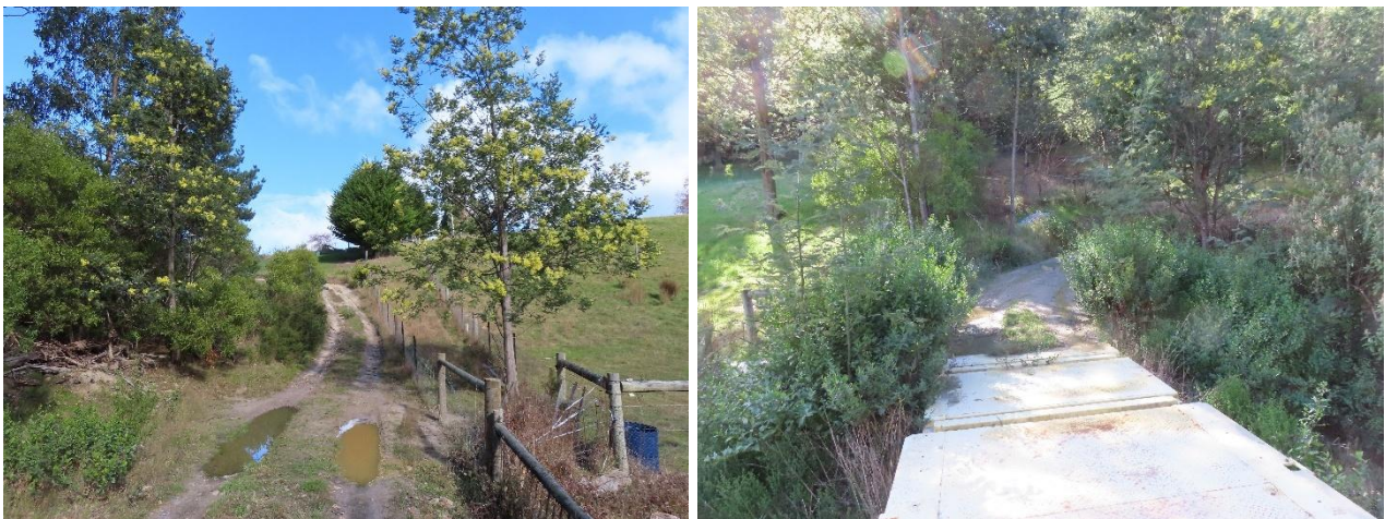
Plates 13 & 14. Southern (LHS) and northern (RHS) approach to new bridge showing well-formed and well-drained formation with no evidence of sediment input into Bates Creek
