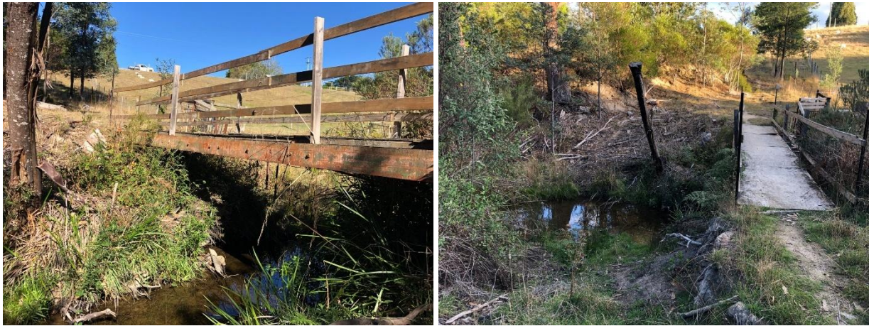
Plate 5. (LHS) Side view of original bridge prior to works – note that the bypass track went east of (i.e. to left of image) the dead Acacia dealbata tree shown in image (this tree was naturally windthrown prior to bridge replacement) [© C. Weir]
