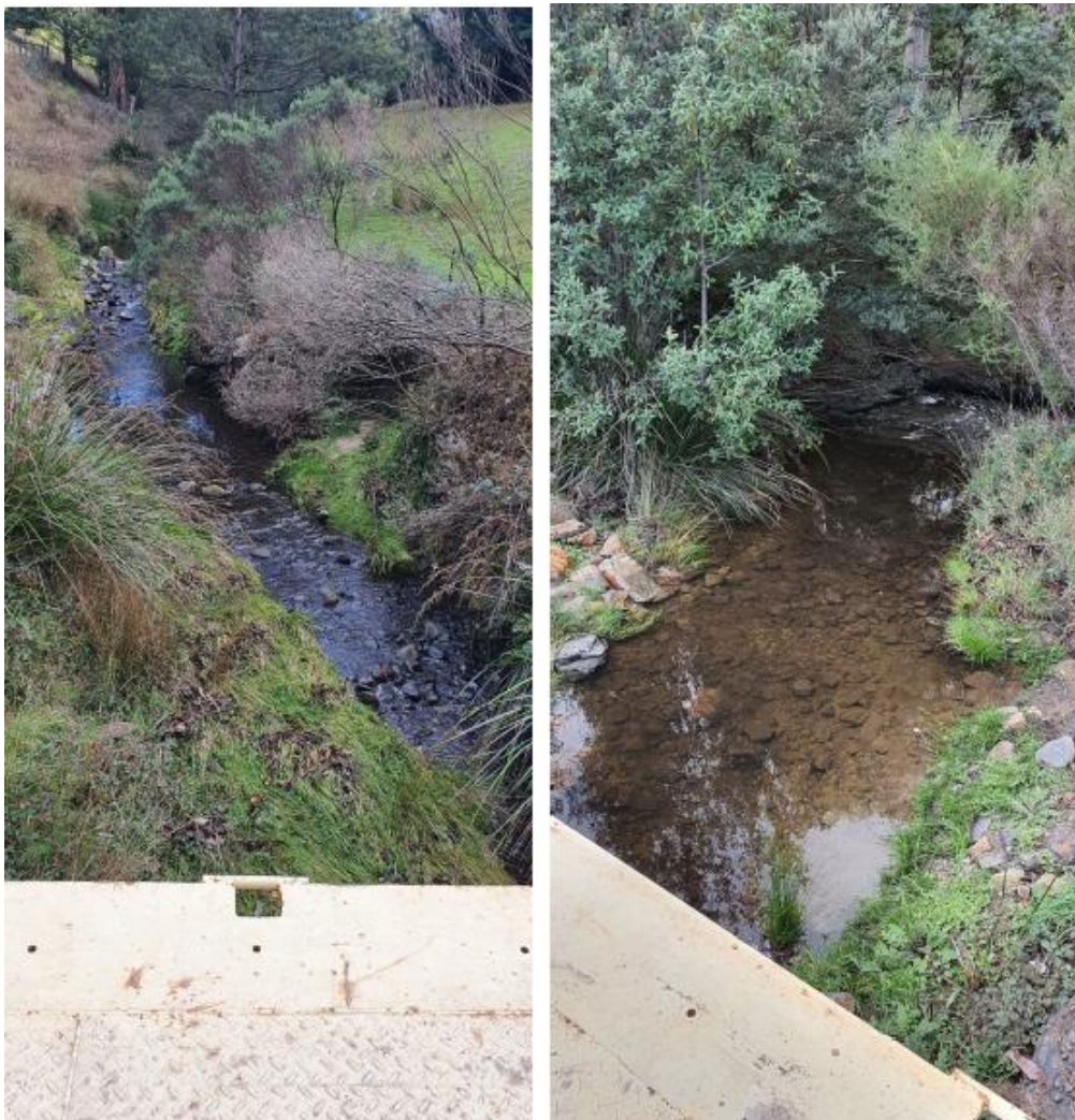
Plates 9 & 10. Views upstream (LHS) and downstream (RHS) of Bates Creek after installation of new bridge and provision of rock "rip-rap" showing no impact to the bed and banks (apart from the small area of "rip-rap") of the creek on either side and no impact to native vegetation [© C. Weir]
