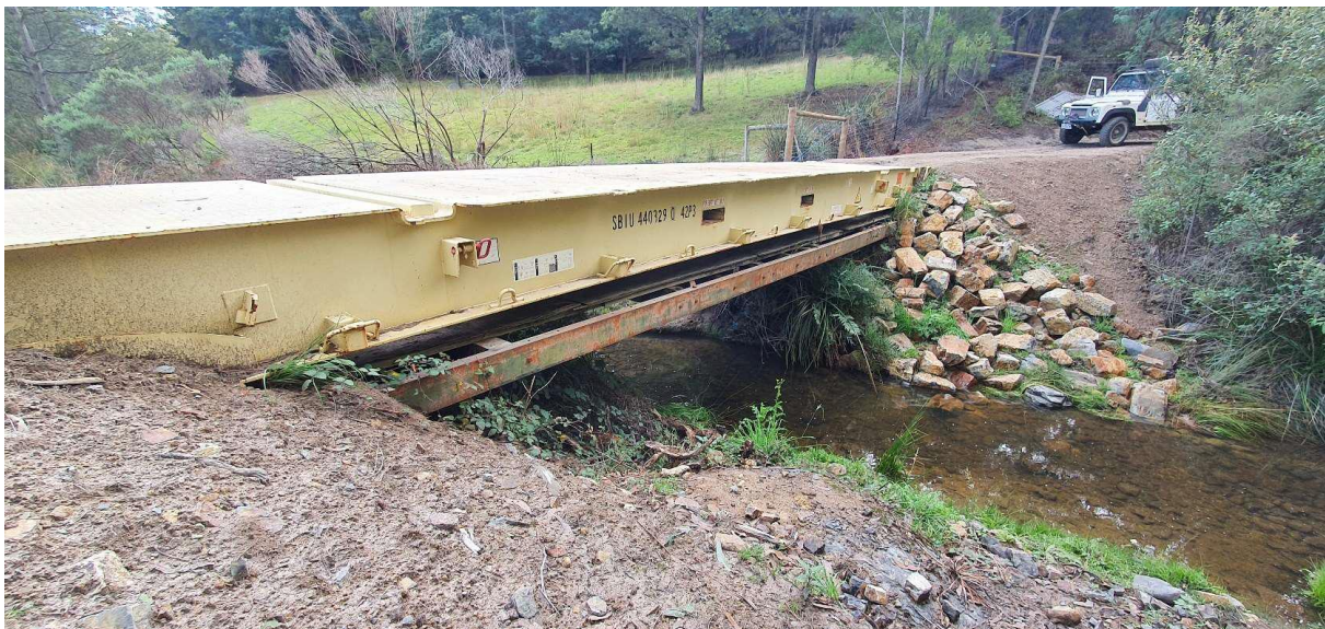
Plate 7. View of new bridge (view from southeast side) showing container base over the top of the original structure, minor shaping of soil profile to facilitate entry/exit and placement of dolerite "rip-rap" on northern side [© C. Weir]
