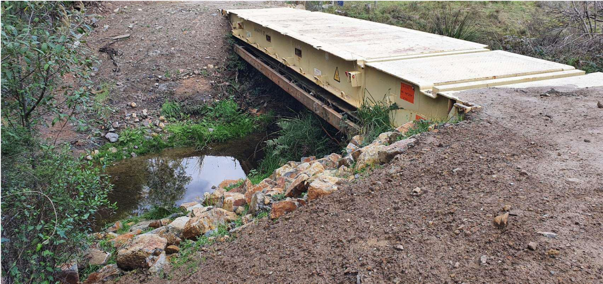
Plate 8. View of new bridge (views from northeast side) showing container base over the top of the original structure, minor shaping of soil profile to facilitate entry/exit and placement of dolerite "rip-rap" on northern side [© C. Weir]
